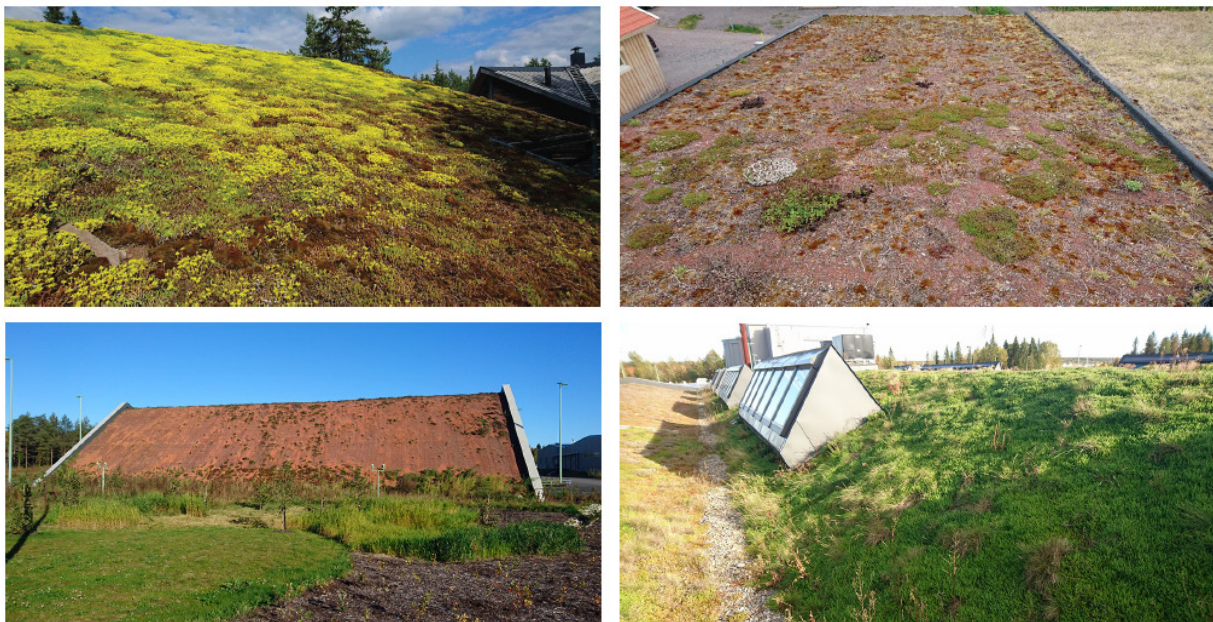
Figure 17. Green roofs with different angles and high and low vegetation coverage illustrating the need for site/climate-specific choice of vegetation.
