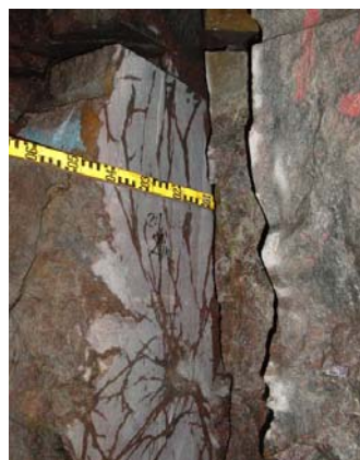
Cracks around water-filled hole
