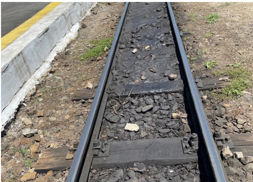
Figure 3. Considerable leaching of diesel and oil from locomotive operation
